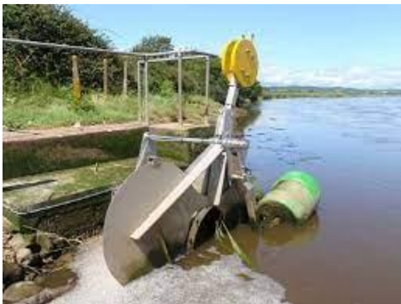
Plate 5 Self regulating tide gate at Seaton in Devon (Figure 3.6 in https://assets.publishing.service.gov.uk/media/6033a8f5e90e076607c1bf0e/Self-regulating_tide-gate_a_new_design_for_habitat_creation_technical_report.pdf )
